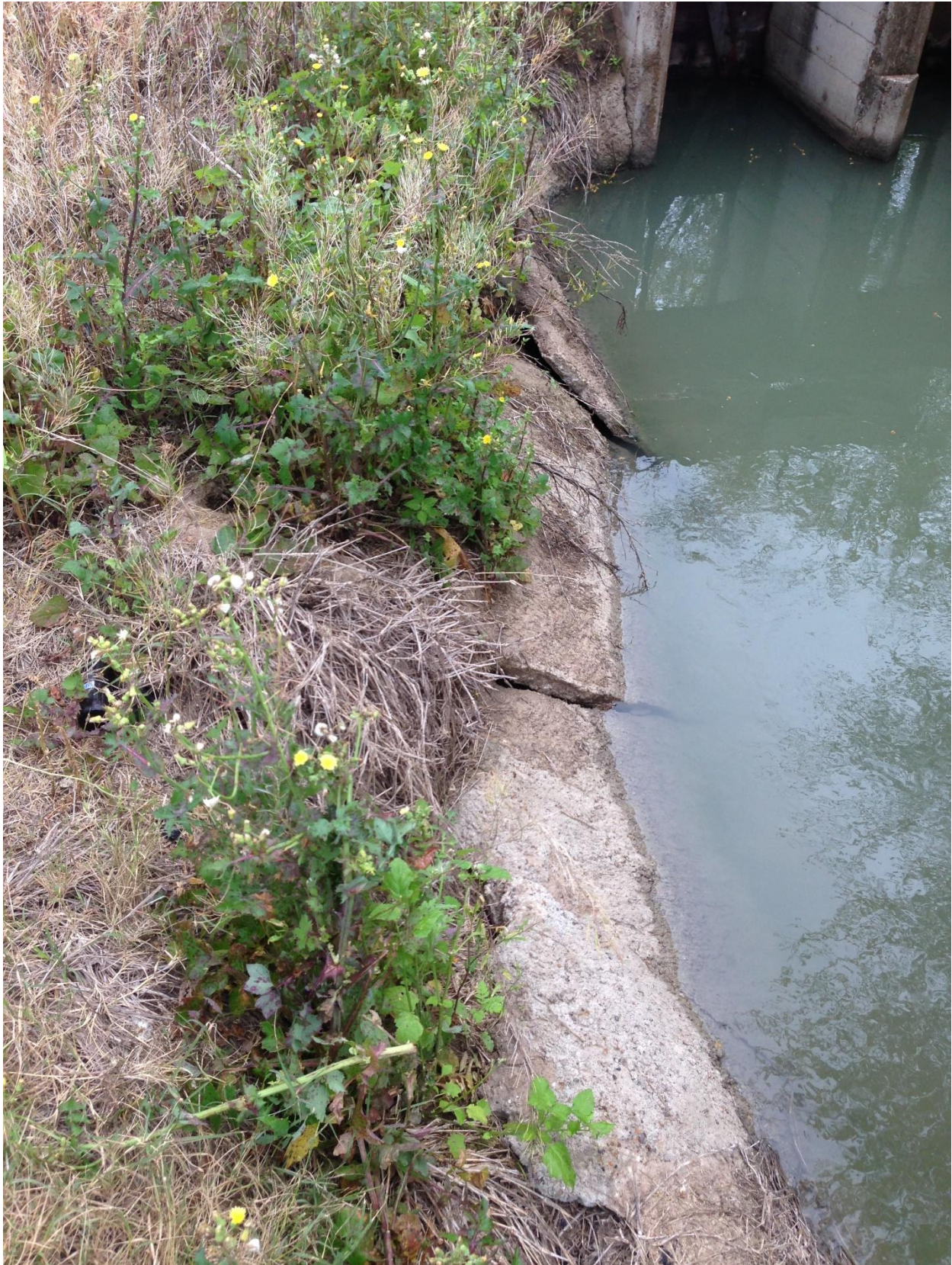
Figure 4 Photograph of dilapidated liner.
